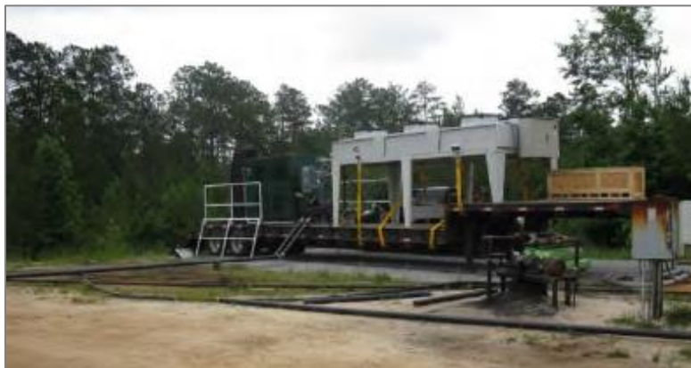
Figure 2. Trailer mounted Green Machine on site in Mississippi for Demo on an oil well.
