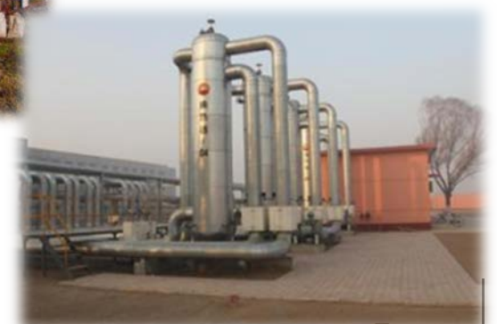
Heat exchanger and geothermal power generation plant (Huabei oilfield, China)
