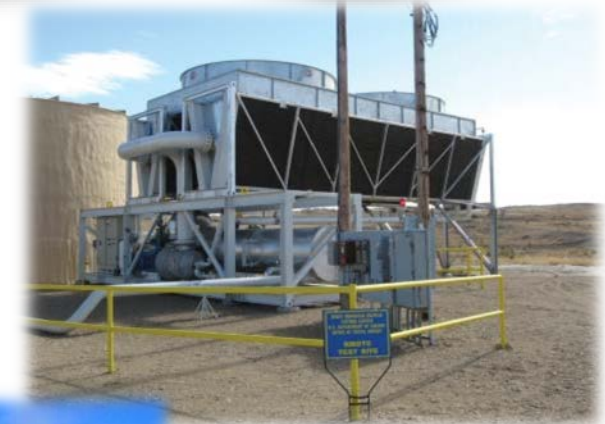
Ormat Organic Rankine Cycle (ORC) 250 kW, Rocky Mountain Oilfield Testing
