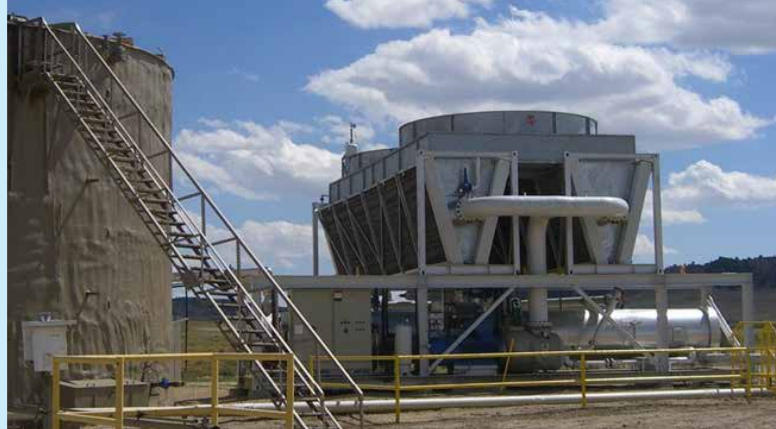
Air-cooled unit on test at Rocky Mountain Oilfield Testing Center.
