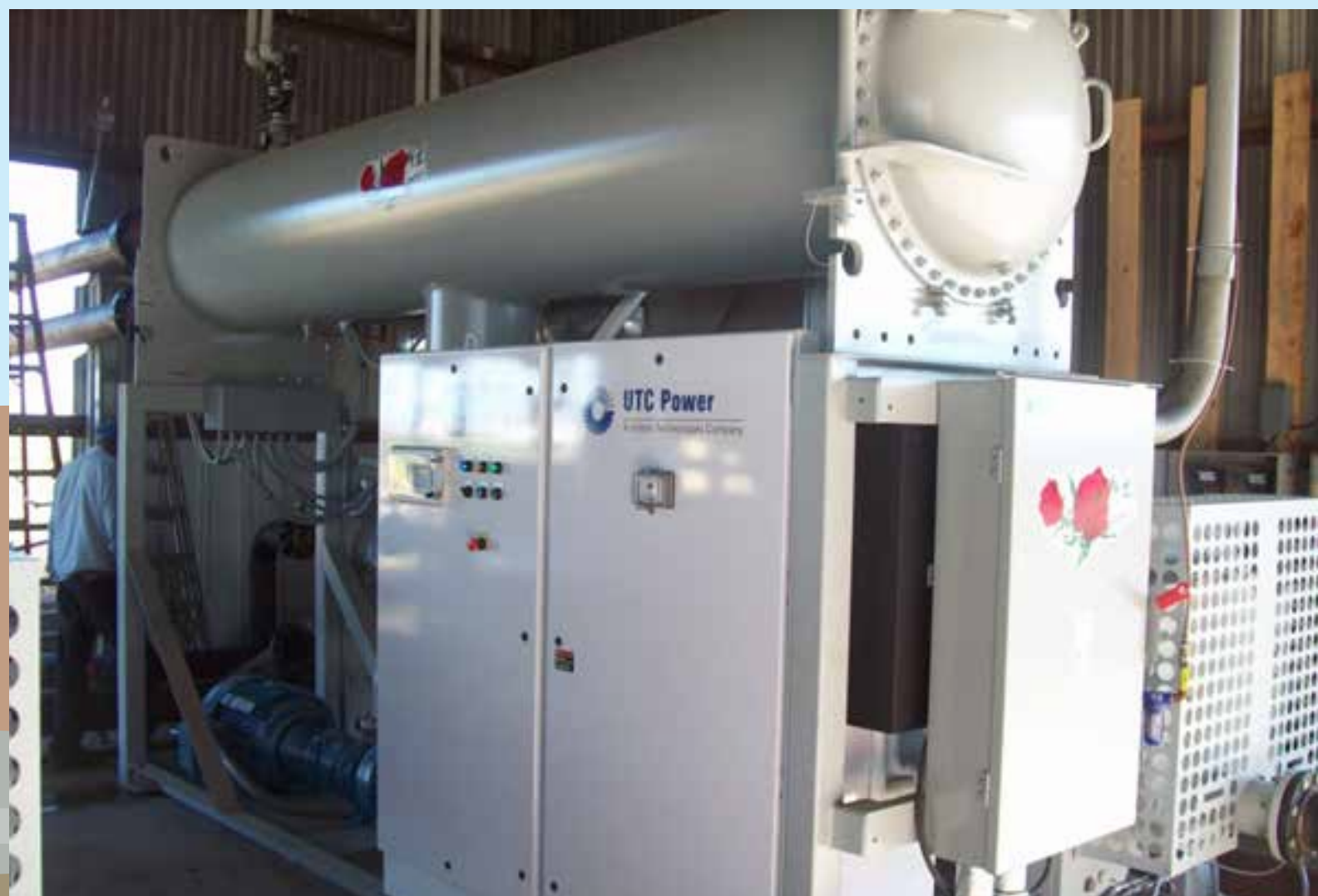
Water-cooled unit in operation.
