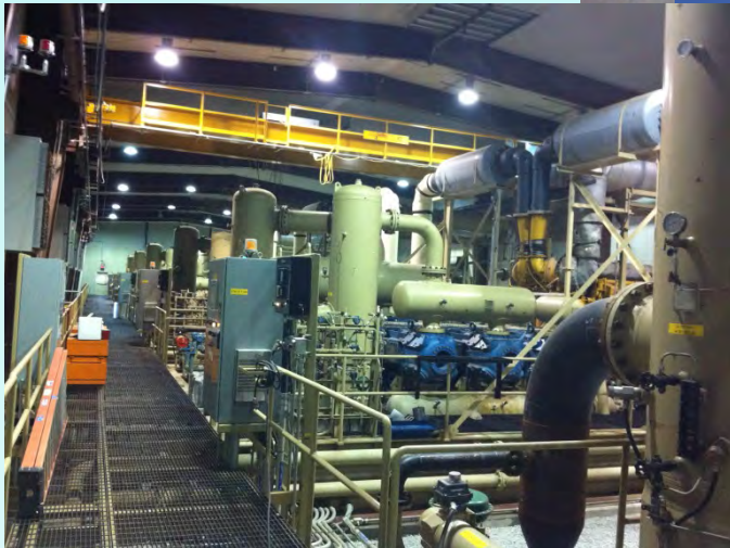
Compressed Gas Cooling
