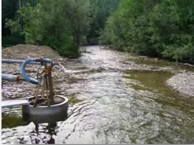
Monument Creek Provides Cooling Water (~40F)
