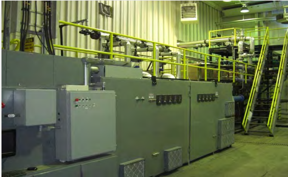
Front view of heavy duty electronics cabinets.
