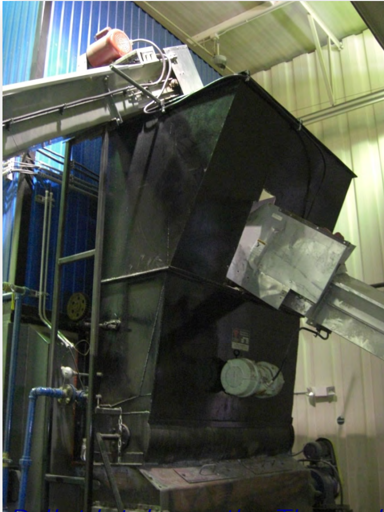
Pellet intake on the Thermal Oil Heater.
