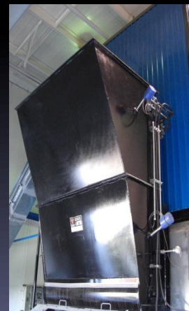
Boiler fuel intake
