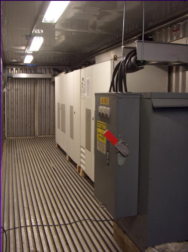
UPS System (MGE)
