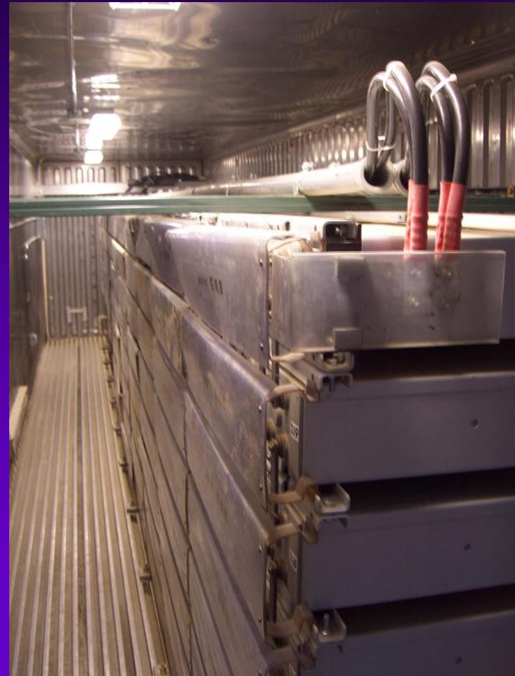
Batteries 3MW Total
