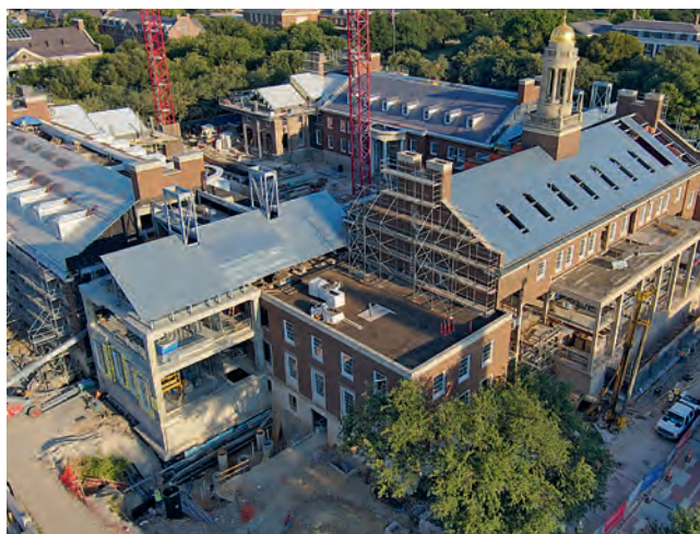
Cox renovations – SMU broke ground on a $140 million renovation and expansion project designed to train students for a collaborative and technologically integrated world.
